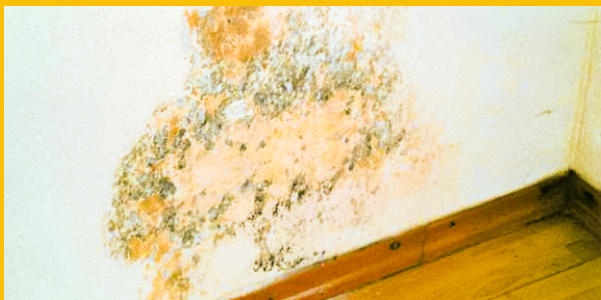
This mould formed behind a wardrobe on an existing wall.
