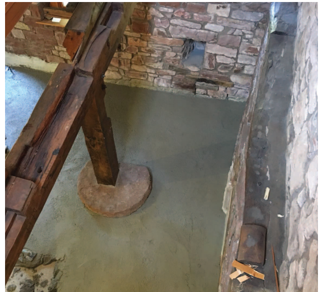
Above, 50mm of Diathonite Cork Lime Screed was applied to the existing concrete floor
