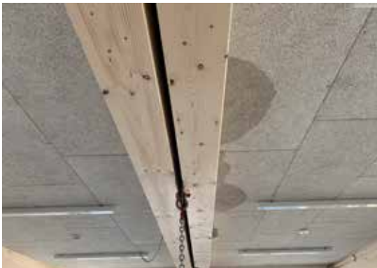
Leaky module joint
