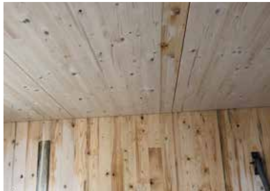
Ugly water stains on a cross-laminated timber ceiling
